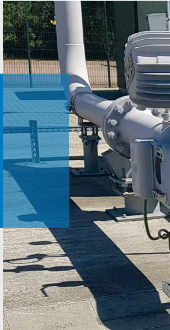
Split body control ball valve at VNG underground gas storage site
