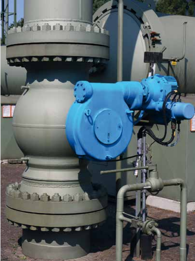
Fully welded ball valve at Thyssengas gas compressor station
