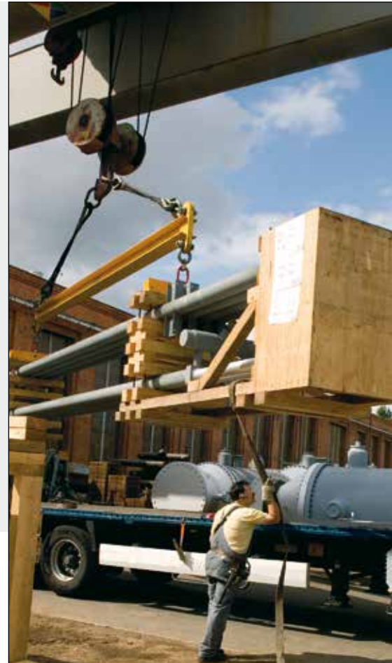
Transfer Line Exchangers at the works area
