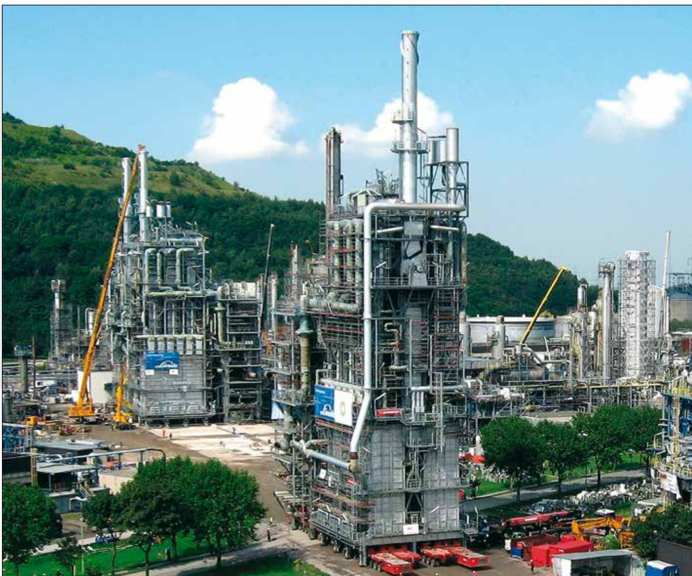
Naphtha Cracking Furnaces
