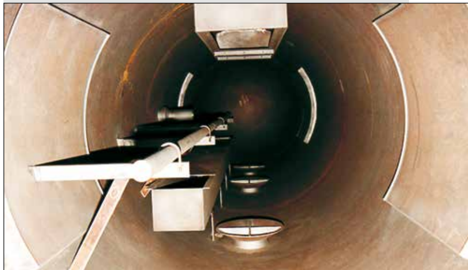
Steam drum internals
