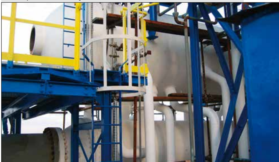
Secondary Transfer Line Exchanger / Steam Drum Unit
