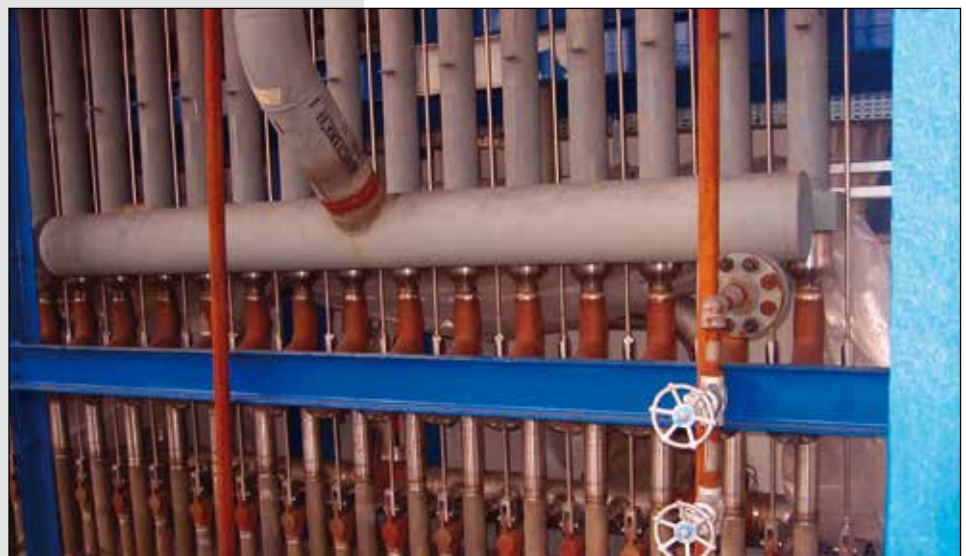
BLQ in the furnace structure
